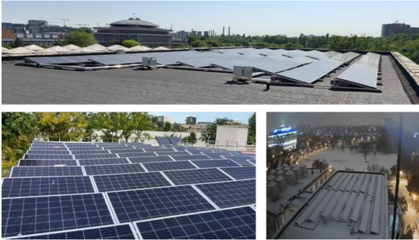
Figure 79. PV system at the Faculty of Power Engineering in NUSTPB.
