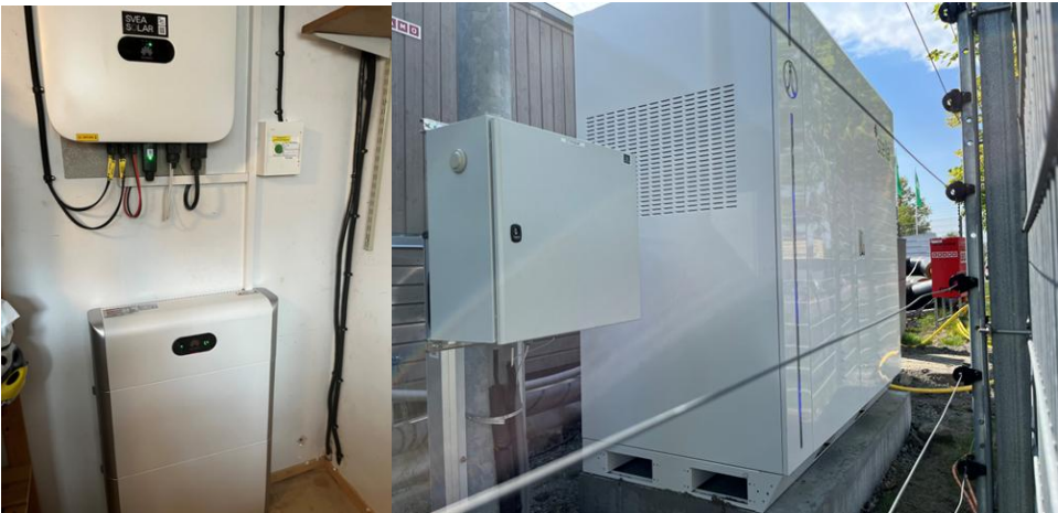
Figure 86. Swedish demo site. Residential battery with inverter (left) and a Commercial & industrial battery installation (right)
