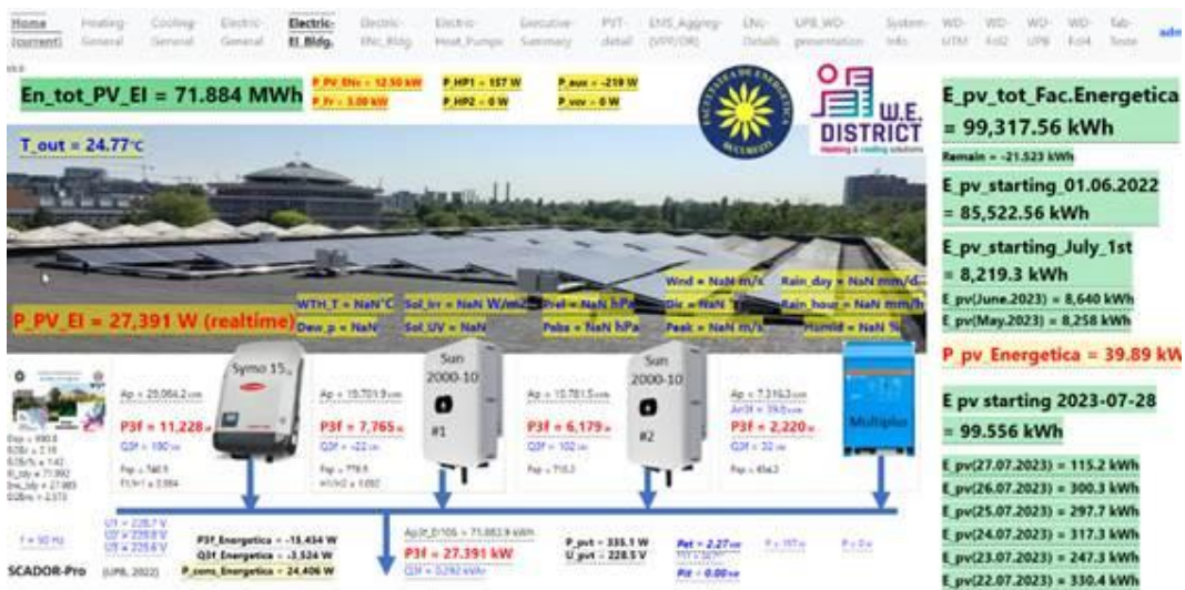
Figure 80. Main PV system in NUSTPB (40 kW).
